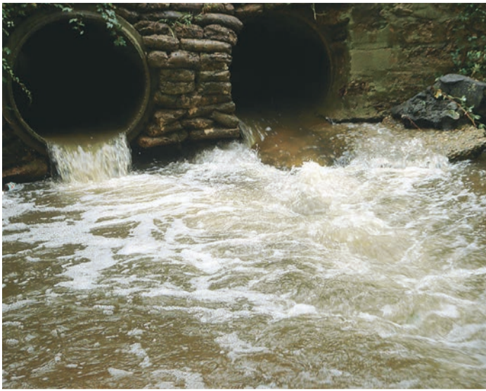
Stormwater flowing from an outfall in Paul Spring Creek in the Mount Vernon area during a storm.
